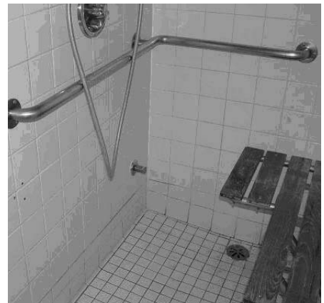
Figure 1. Steam shower seat area (outlet pipe indicated)
